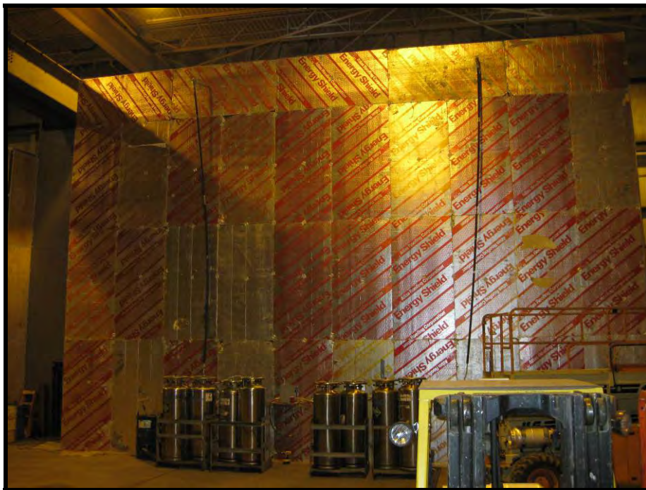
Photo No. 4 Exterior View during Thermal Cycling
